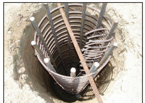
Caissons A wire cage, with reinforced steel bars, is lowered into a pre-drilled caisson hole. Concrete is then poured in and around the cage to create a strong support pillar. The foundation of the new wing will be supported by 32 of these caissons, each about 30 to 60 inches in diameter and 10 to 15 metres deep.
